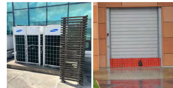
Rooftop Outdoor Unit and Facility Anchoring
