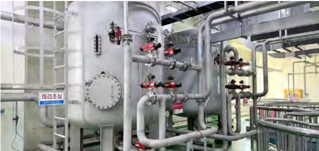
Celltrion Pharm Wastewater Treatment Plant
