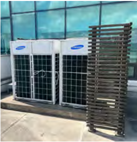
Rooftop Outdoor Unit and Facility Anchoring
